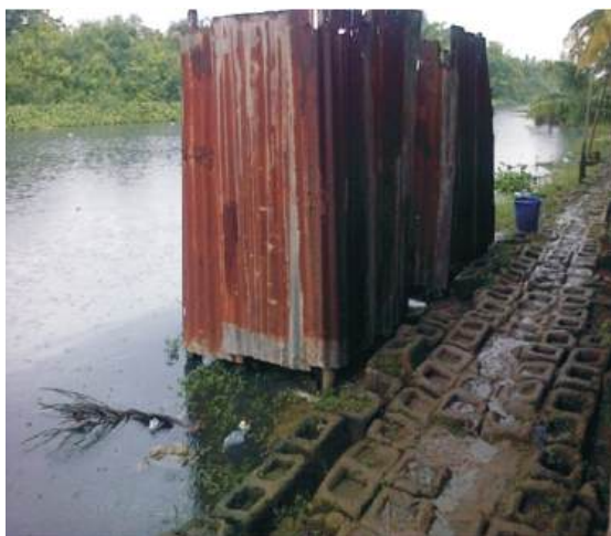
Figure 3: Toilet and bathroom built on a river
