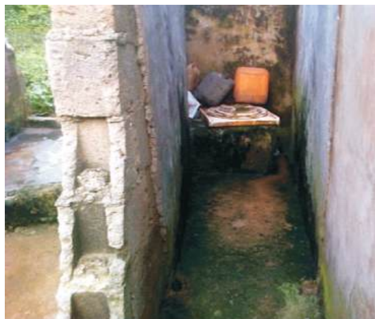
Figure 5: An abandoned toilet
