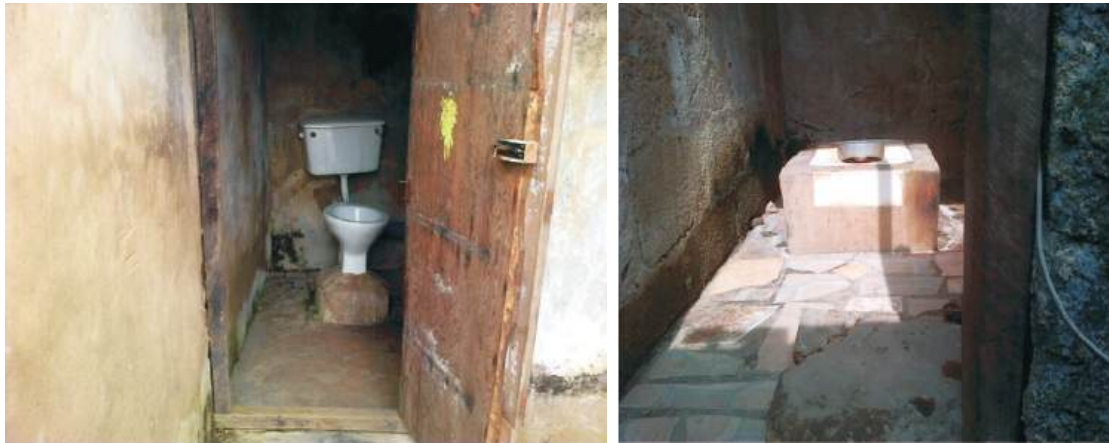
Figures 2a and b: Toilet facilities in some of the houses
