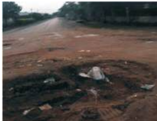
Plate 23: Estate road eroded by rainwater
