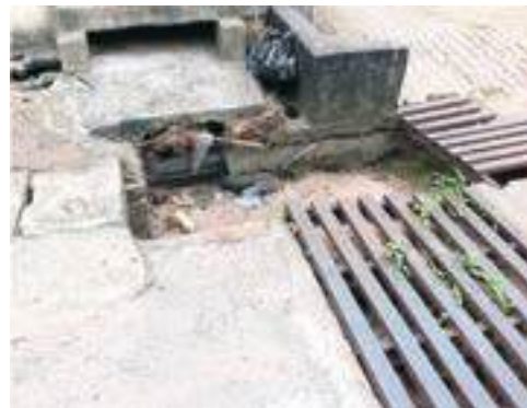
Plate 13: Blocked and broken drain
