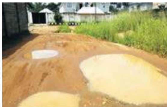
Plate 31: Potholes on the road
