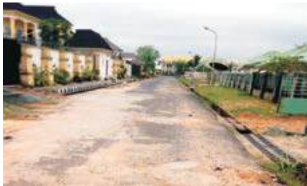
Plate 12: Road showing patched up areas
