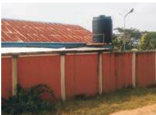
Plate 6: Overhead tank for water storage
