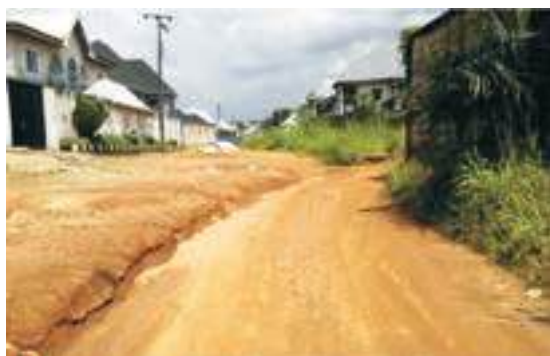
Plate 30: Road badly eroded by water
